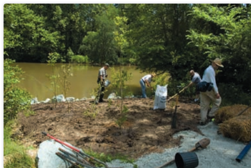
Repairs are made to an eroded section of the Haw River shoreline at Jordan Lake State Recreation Area.
