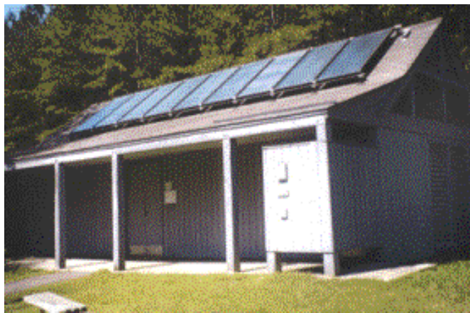
Solar-powered shower house - Energy Efficiency
